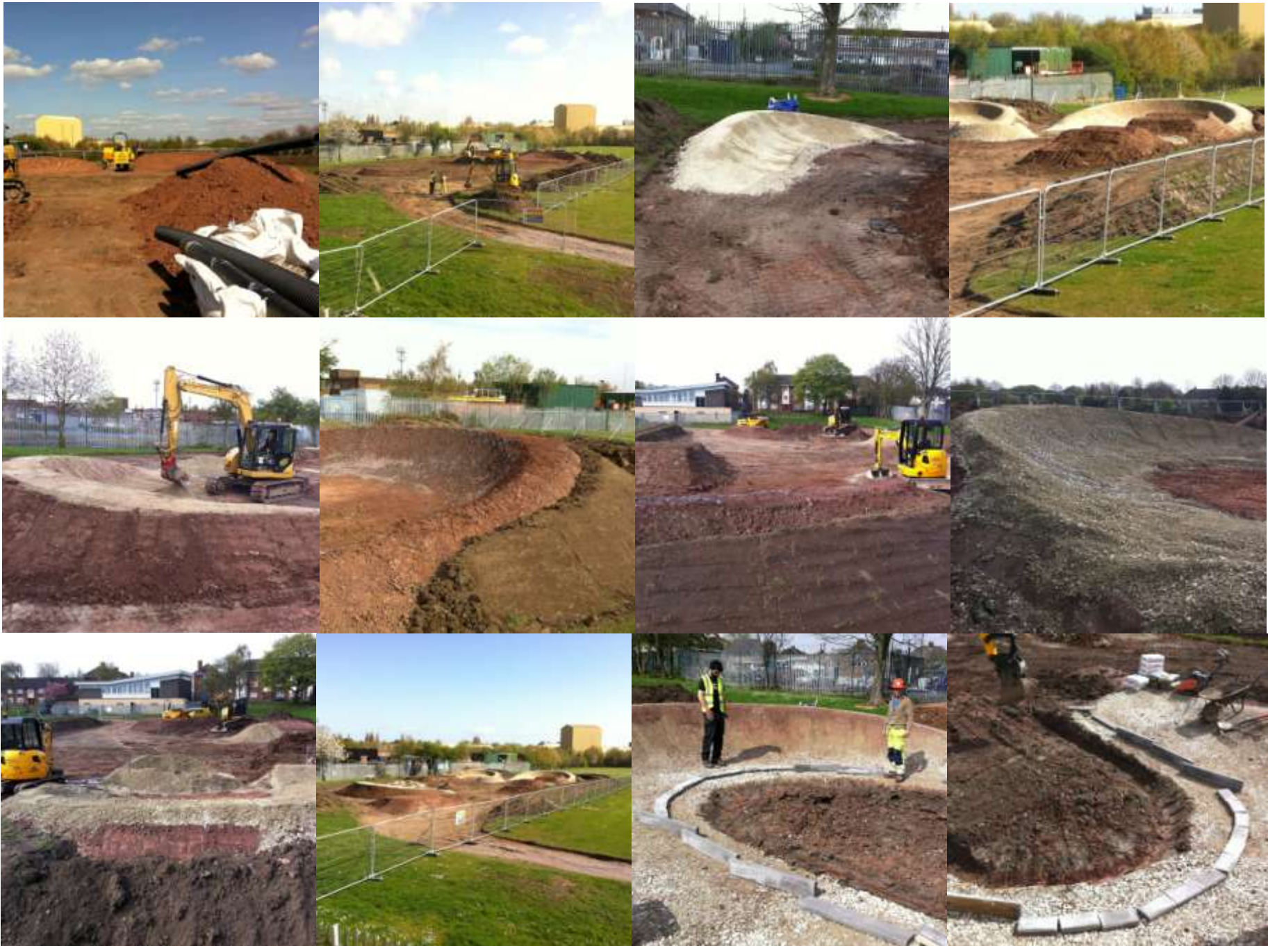
James, Shaun & Nikki started construction work on our New BMX Cycle Track on Thursday 10th April 2014 & these photos show the progress of the build
